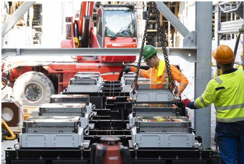
The last transformer is lifted by crane and placed and aligned with millimeter precision at the demonstration plant.
